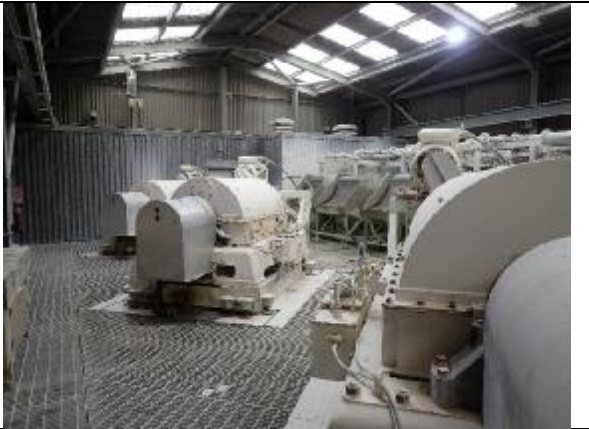
Centrifuges in the clay processing plant
